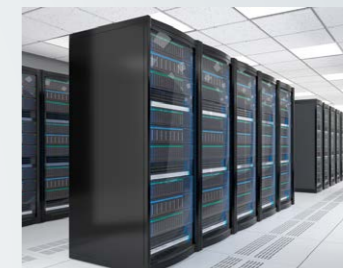
Data centers that support high-capacity communication
