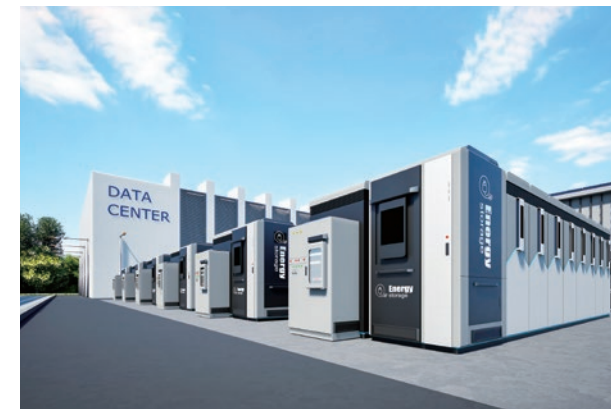
Many ESS units are installed in data centers
