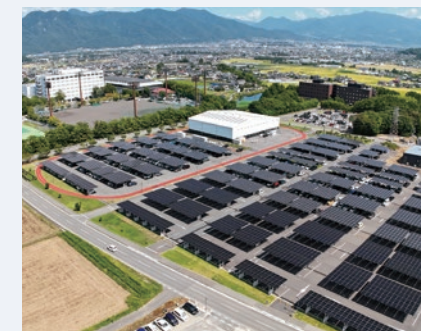
Solar carport on the headquarters grounds
