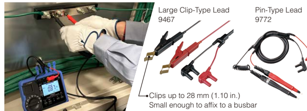
Low-resistance measurement Continuity test after ground resistance measurement
